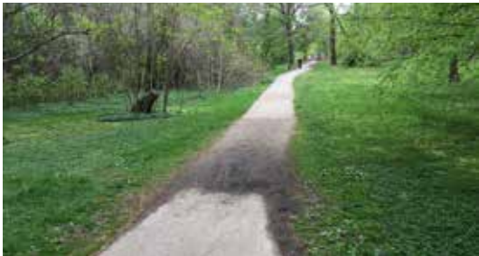
Area of poor drainage in Linkwood Park
