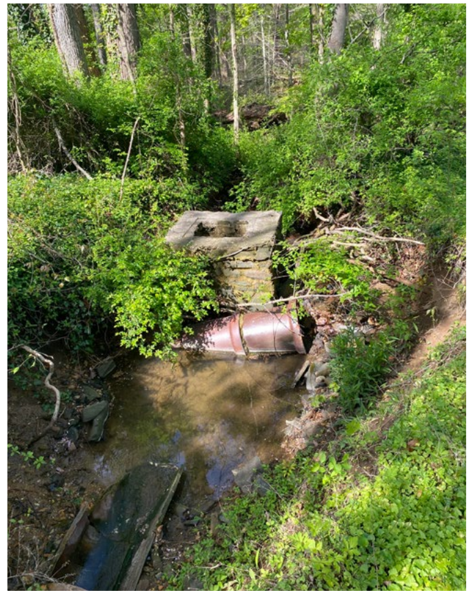
Deteriorating pipes also impact current conditions in the park's streams. Photo: Mary Page Michel
